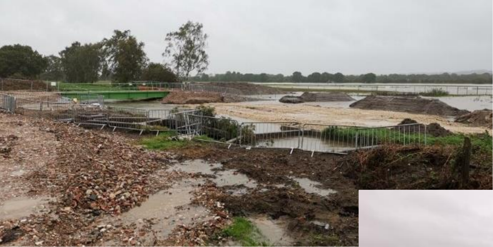
20.10.23 - Boultham Catchwater Breached (Lindum construction site flooded @ Pig Lane)
